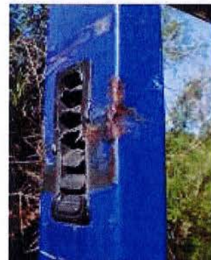
x Unacceptable damage to overhead guard
