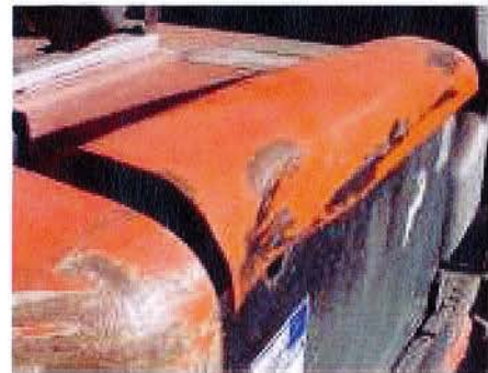
x Unacceptable dents to a battery cover
